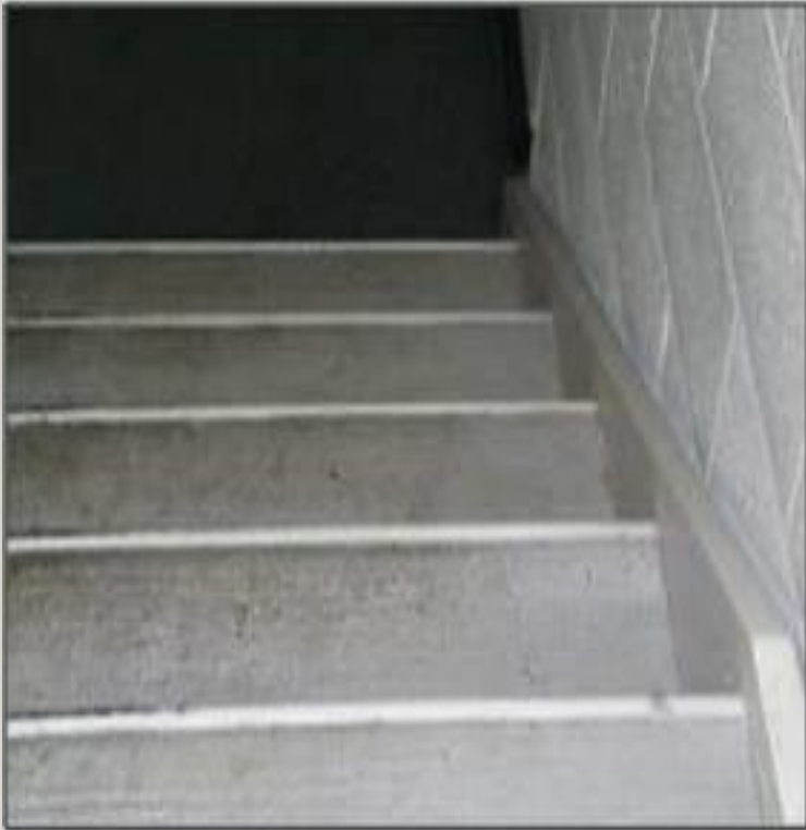
Non-slip threads on stair edges
